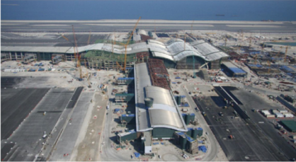
NDIA Airport, Doha
